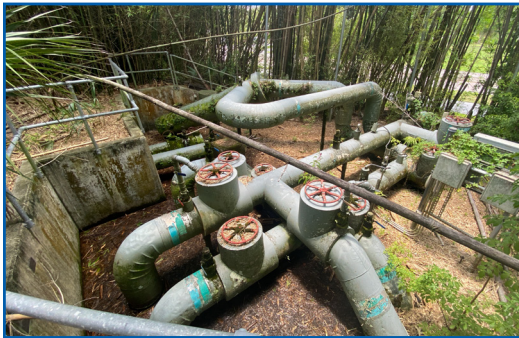
Polynesian Resort Chiller
